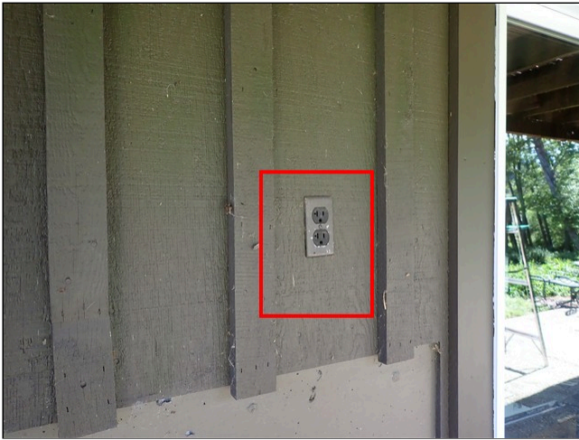
2.5 ELECTRIC / GFCI (Picture 1)
