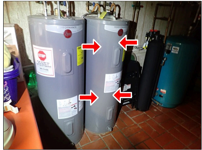
13.2 WATER HEATER 2 (Picture 2)
