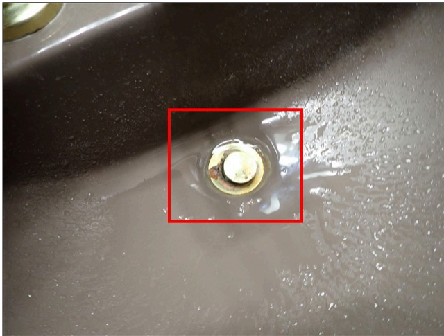
7.1.A SINK(S) (Picture 1)
