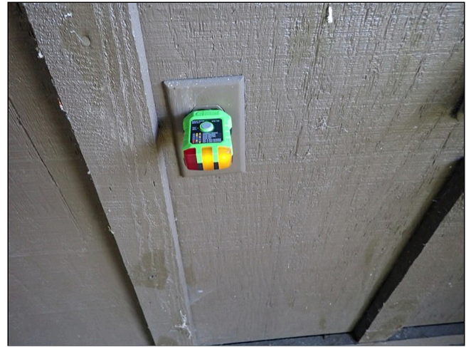
2.5 ELECTRIC / GFCI (Picture 2)
