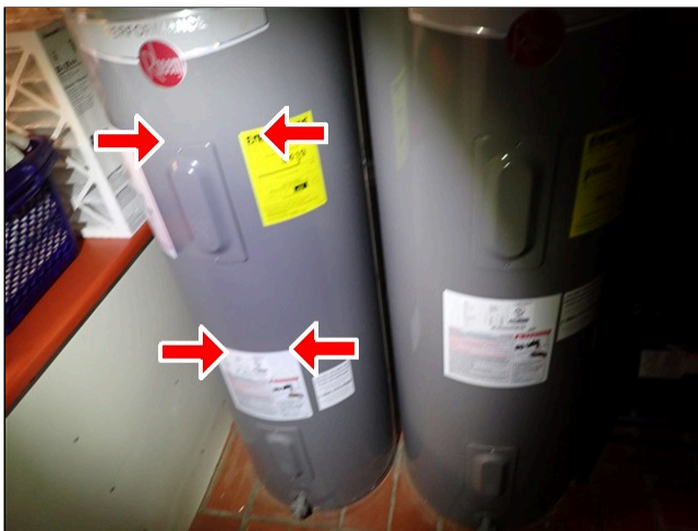
13.0 WATER HEATER 1 (Picture 1)
