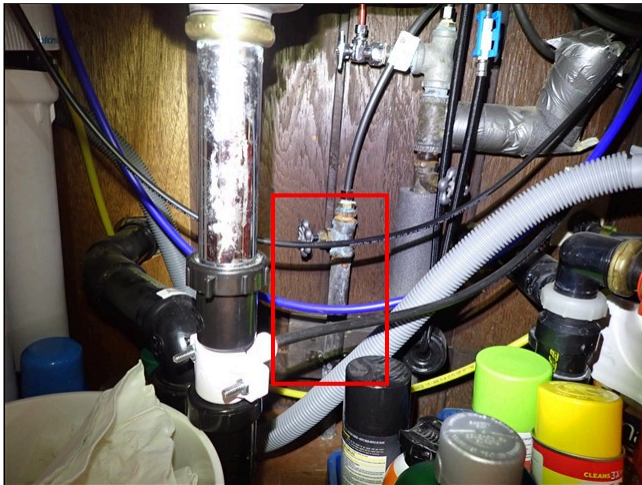
12.0 WATER SUPPLY PIPING (Picture 1)
