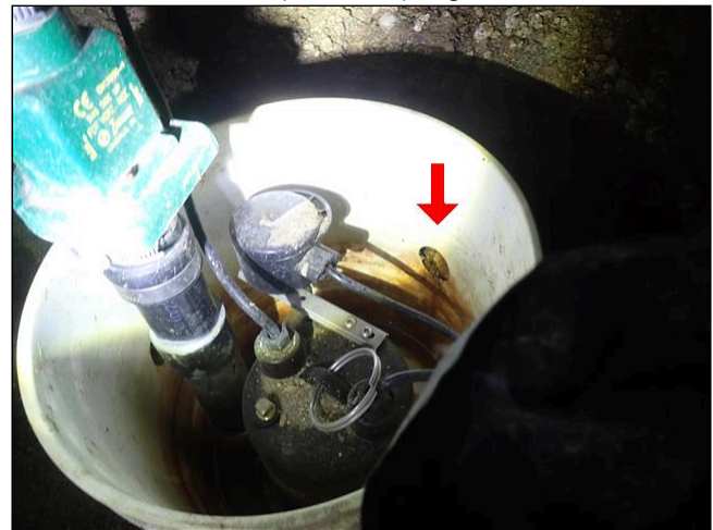
10.2 SUMP PUMP (Picture 2)
