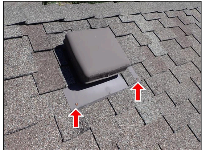
1.4 VENTILATION COVERS (Picture 1)
