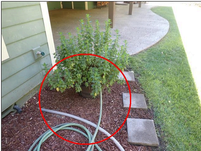
10.2 SUMP PUMP (Picture 3)
