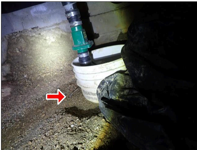
10.2 SUMP PUMP (Picture 1)
