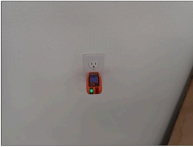
4.5 ELECTRIC / GFCI (Picture 1)
