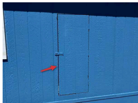
Water Heater Door
