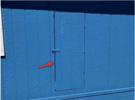
Water Heater Door
