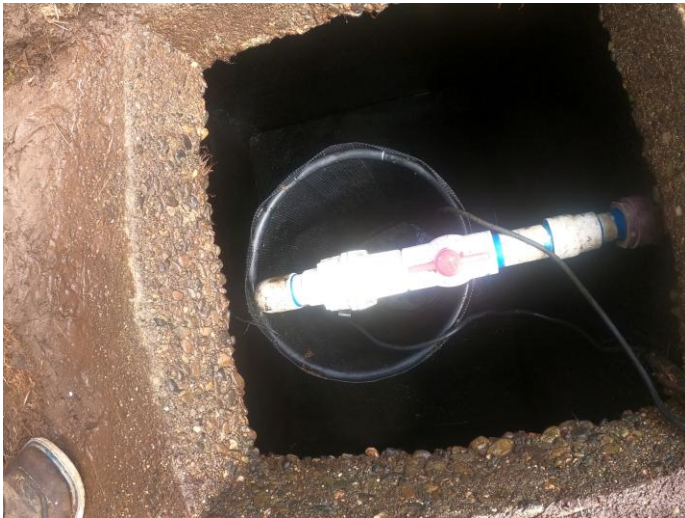
Dosing Tank / Pump System
