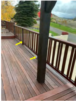
South railings loose
