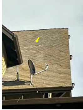
Patch on west side
