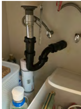
No sign of leaking under upstairs guest bath sink at this time
