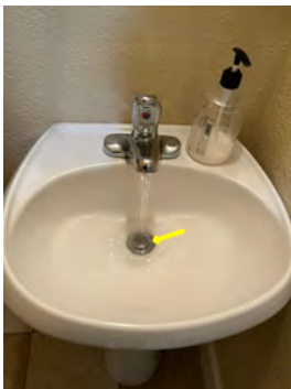
Stopper not connected in basement 1/2 bath
