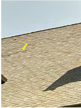
Patch on west side
