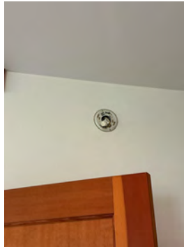
North guest bedroom missing smoke detector recommend installing unit
