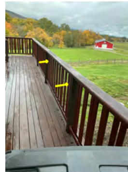
North railing loose
