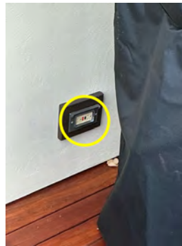
Missing GFCI cover on west outlet on patio
