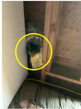
North end of attic bath fan vented into attic, recommend this be vented to the exterior
