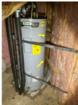
need blocks behind water heater to make unit solid so does not move in a earthquake
