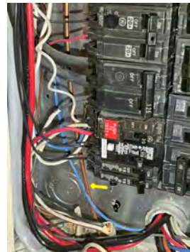
Panel A Copper Ground wire
