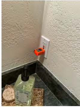
Laundry bathroom GFCI works good
