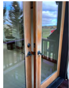
Finish wearing thin on master deck doors
