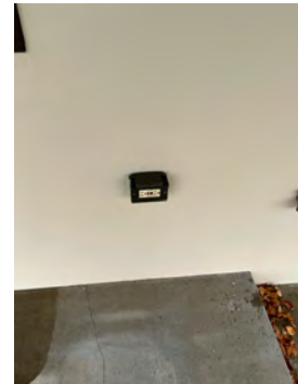
Missing GFCI cover on downstairs west exterior outlet
