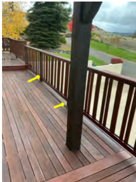
South railings loose
