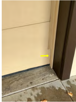
Damaged garage door seal bottom right side
