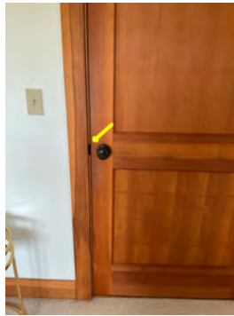
North guest door needs catch adjusted to latch when closed
