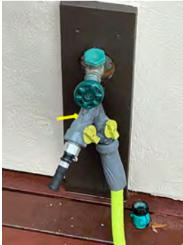
North hose bib leaks, repair or replace
