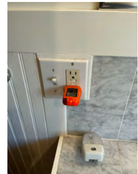
Upstairs guest bath GFCI works good
