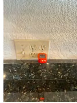
Kitchen GFCI works good
