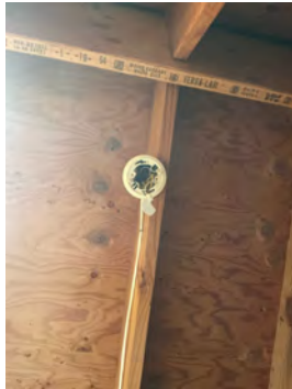
smoke detector in attic space needs to be replaced
