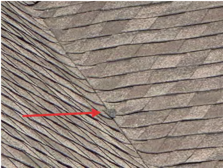
Broken shingle tab in valley.
