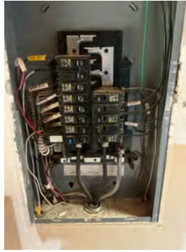
Attic sub panel in good shape
