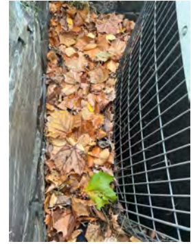
Recommend cleaning the leaves out from around the cooling units
