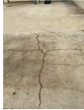
a few small cracks in driveway normal for age of home
