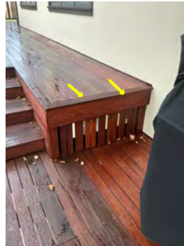
possible fall hazard on west end of the deck, recommend scooting BBQ closer or installing handrail
