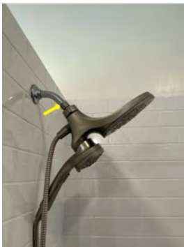
Shower head leaks in upstairs guest bathroom
