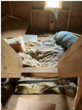
batt insulation in the attic space is adequate
