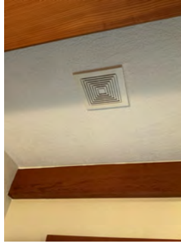
Laundry bathroom fan did not turn on
