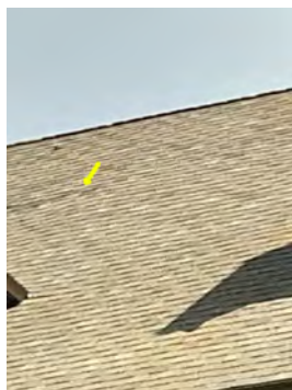
Patch on west side
