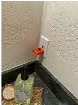
Laundry bathroom GFCI works good
