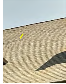
Patch on west side
