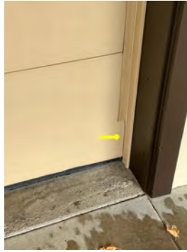
Damaged garage door seal bottom right side
