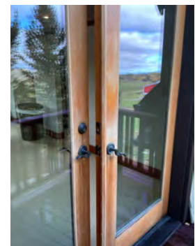
Finish wearing thin on master deck doors
