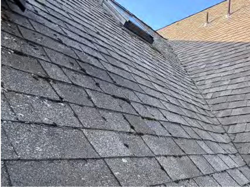
Moss growth on north side of home.
