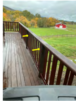
North railing loose
