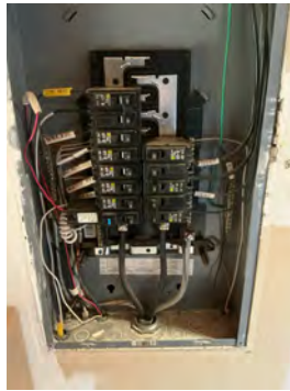
Attic sub panel in good shape
