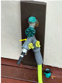
North hose bib leaks, repair or replace
