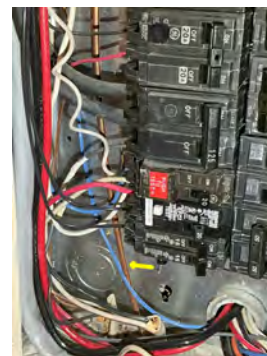
Panel A Copper Ground wire
