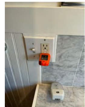
Upstairs guest bath GFCI works good
