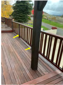
South railings loose
