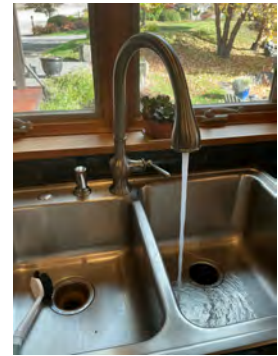
Kitchen faucet works good
