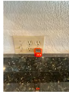
Kitchen GFCI works good
