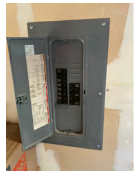
Attic sub panel in good shape
