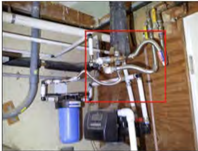
12.0 WATER SUPPLY PIPING (Picture 1)
