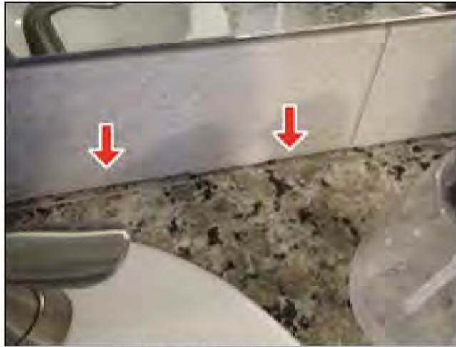
8.0.A SINK(S) (Picture 1)
