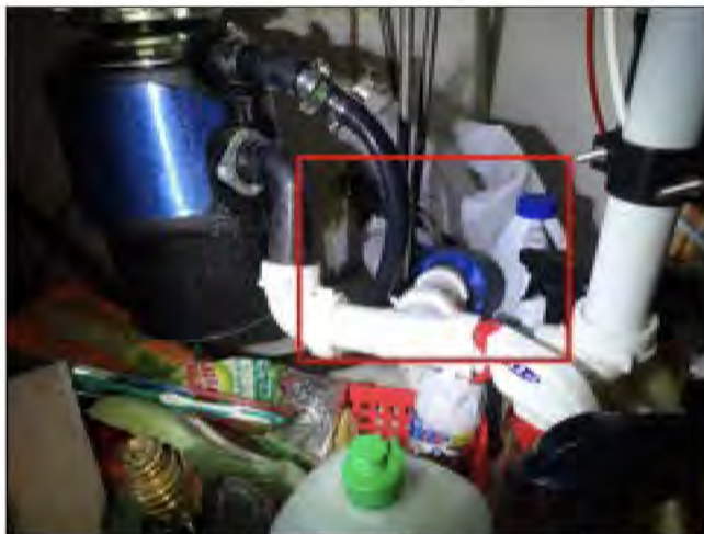
7.0 PLUMBING / SINK (Picture 1)
