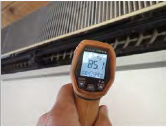
11.3 HEAT PUMP 2 (Picture 1)
