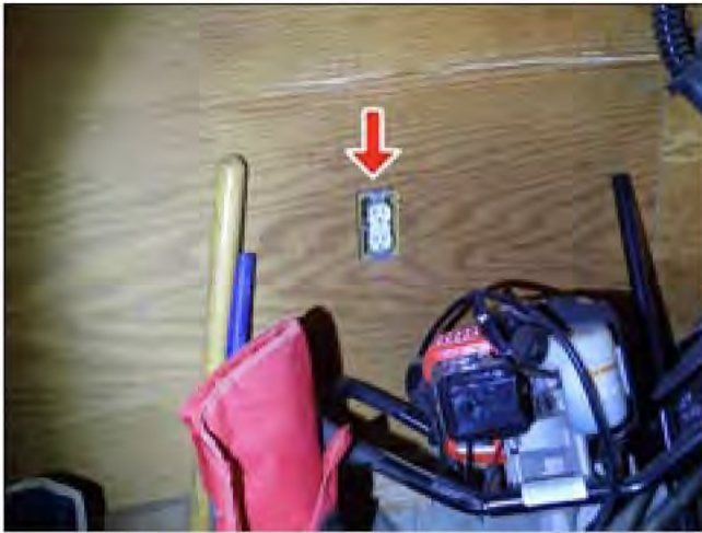
4.5 ELECTRIC / GFCI (Picture 1)
