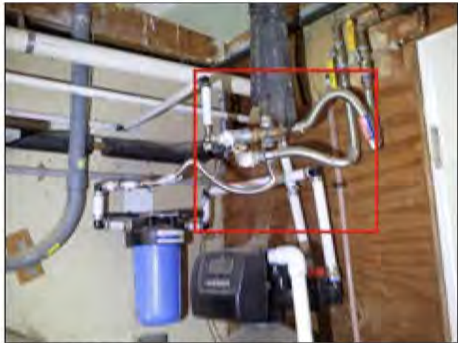
12.0 WATER SUPPLY PIPING (Picture 1)
