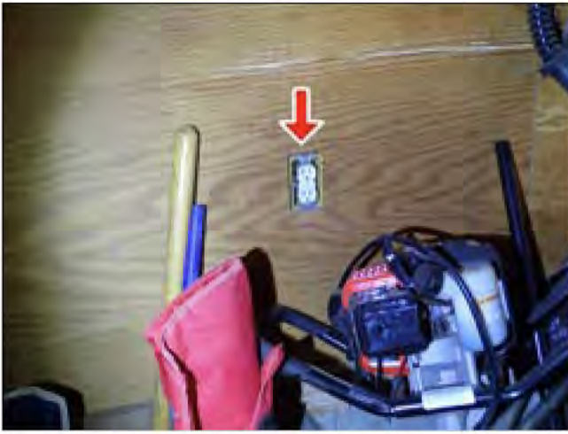
4.5 ELECTRIC / GFCI (Picture 1)
