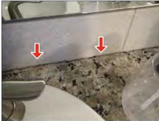
8.0.A SINK(S) (Picture 1)
