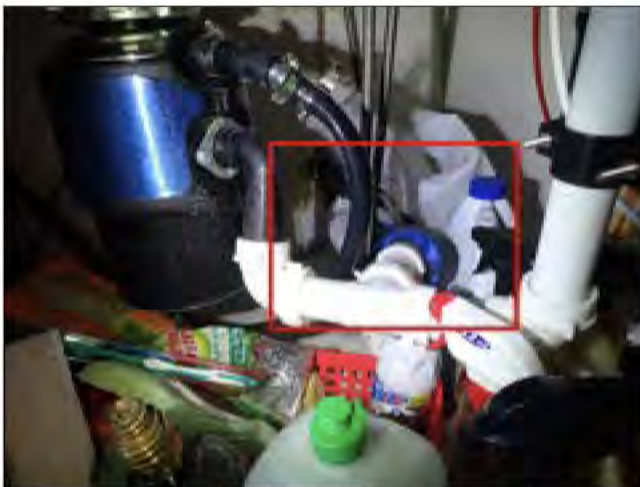
7.0 PLUMBING / SINK (Picture 1)
