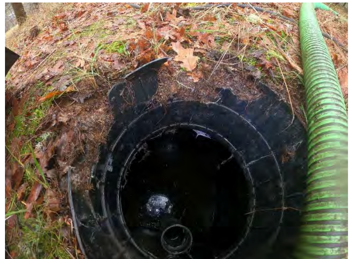
Broken Riser on Outlet side of Tank
