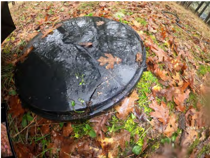
Damaged Lid on Outlet Side
