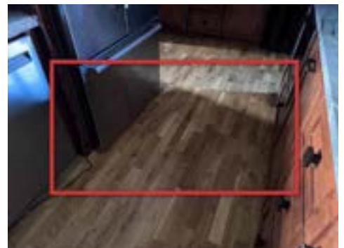
Possible refrigerator or dishwasher leak (dry at time of inspection)
